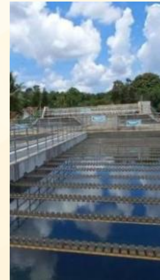
Clean Water System
